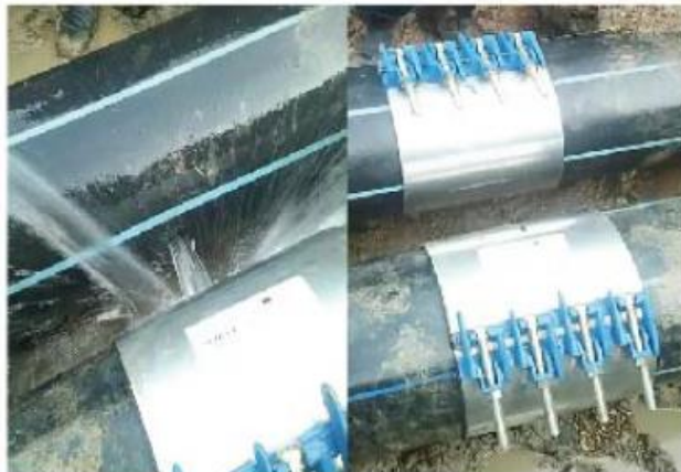
Russian customer use our Repair Clamp of Zhuhong to finish a very fast repairing for the PE pipe of DN300 in water supply.
