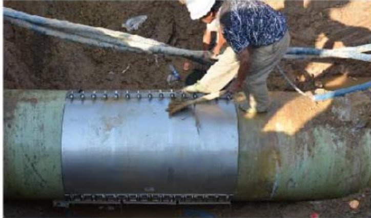
To repair the DN1200 GRP pipe of Hunnan Water Corporation conventionally, they' ll have to stop the water pipe for more than 36 hours. However, using the Repair Clamp of Zhuhong instead just make it within 2 hours.
