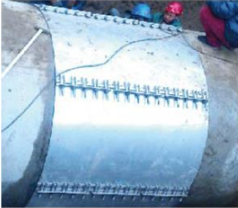
It takes only 3 hours to successfully repair the DN2300 cement pipe with the Band Repair Clamp of Zhuhong.
