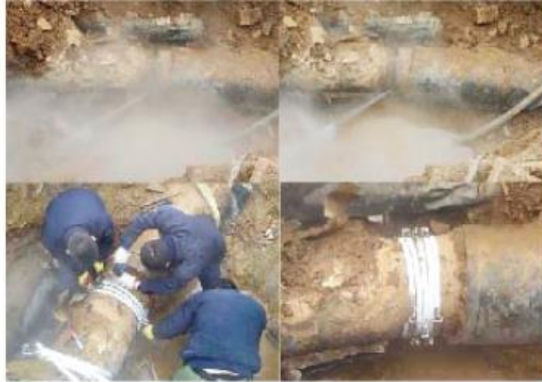
For the leakage of 20° degree elbow of DN450 heating pipe, Zhuhong Elbow Repair Clamps overcome this technical difficulty just in 10 minutes
