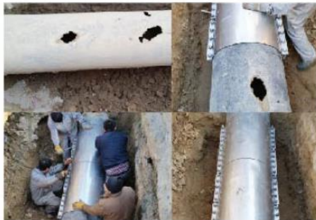
6.Zhuhong Lengthen Type Repair Clamp is used for fast repairing of long leakage of DN900 ductile iron pipeline of Jinan Water Group.
